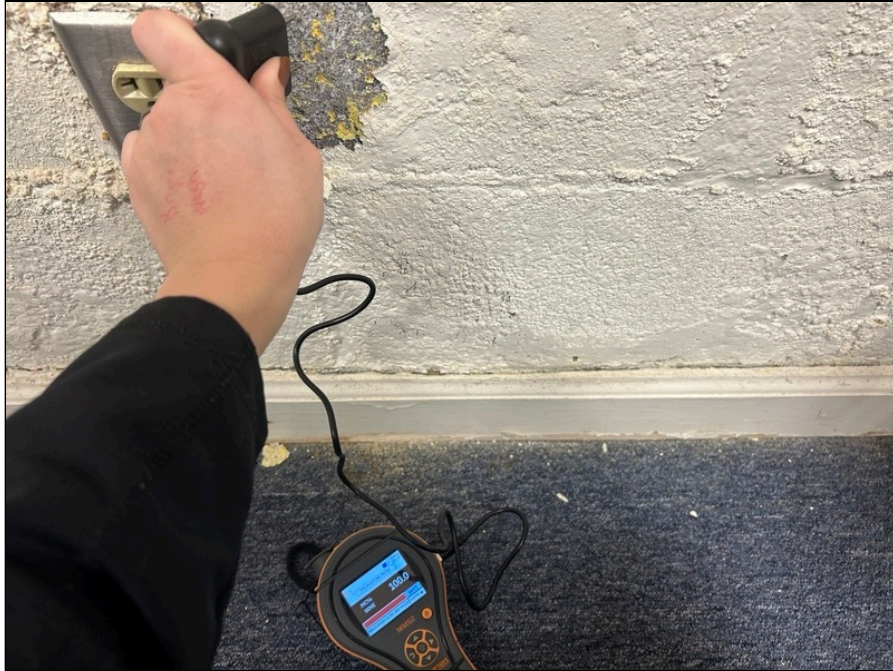
1 - Auditorium Dressing Room - CMU Wall (100% moisture content)
