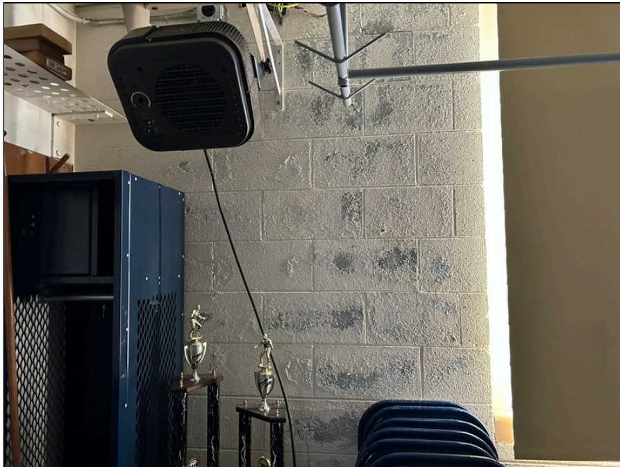
6 - Example of efflorescence on an exterior CMU wall - indicating potential longer term moisture intrusion.
