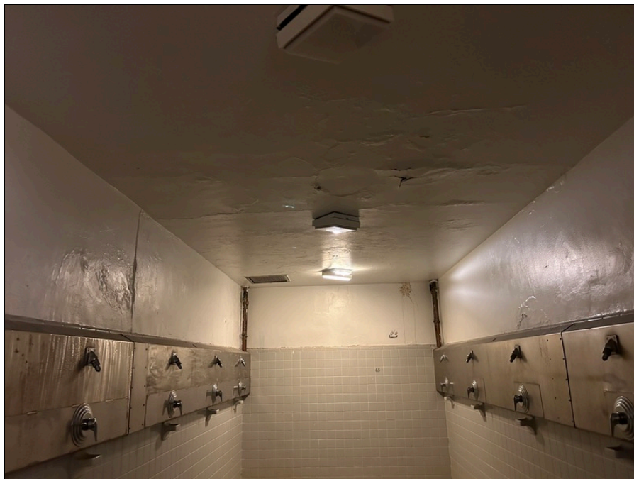
4 - Locker Room Shower with water damaged ceilings; Areas teste dry..
