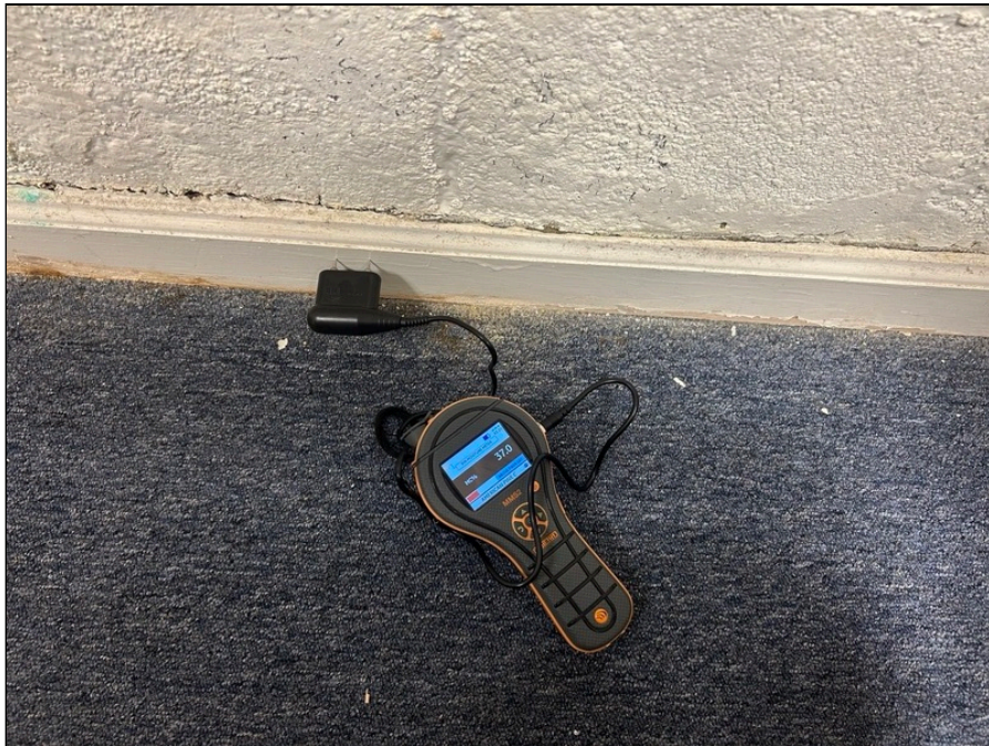
2 - Auditorium Dressing Room - Baseboards Wall (37% moisture content)
