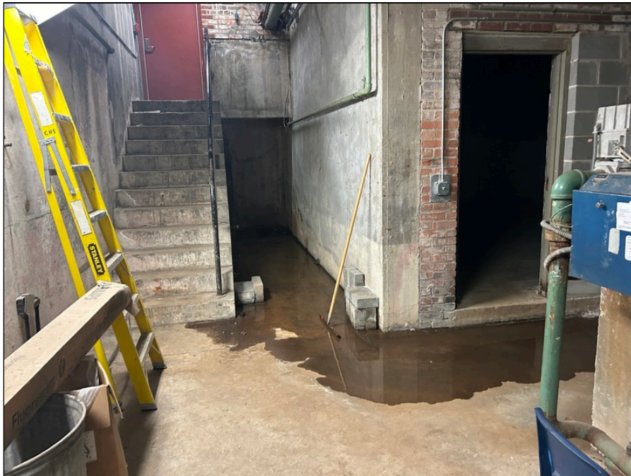
8 - Active water leak in the boiler room for the original school.
