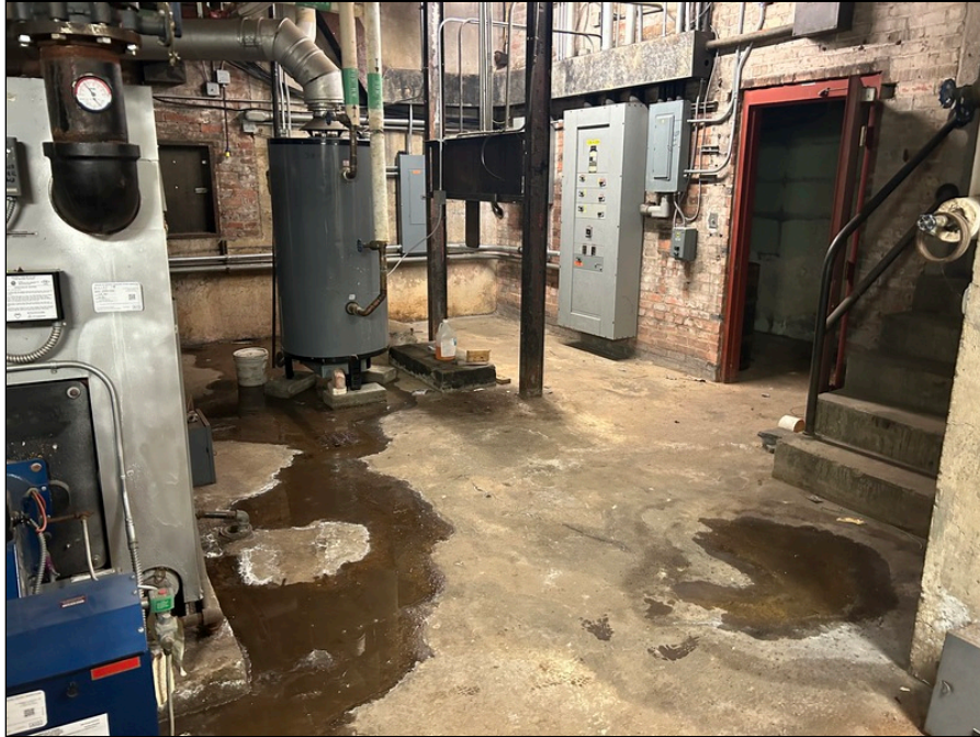
7 - Active water leaks in the boiler room for the original school.
