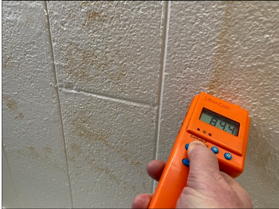
3 - Room 111 CMU Block Wall (84.4% Moisture Content)
