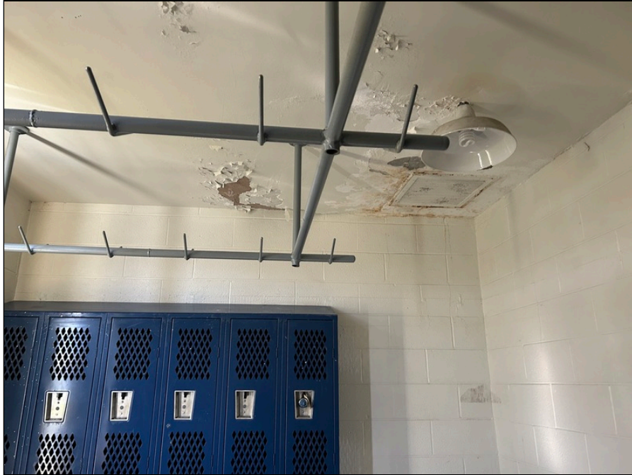
5 - Water damaged ceilings in the locker room area; Areas tested dry.
