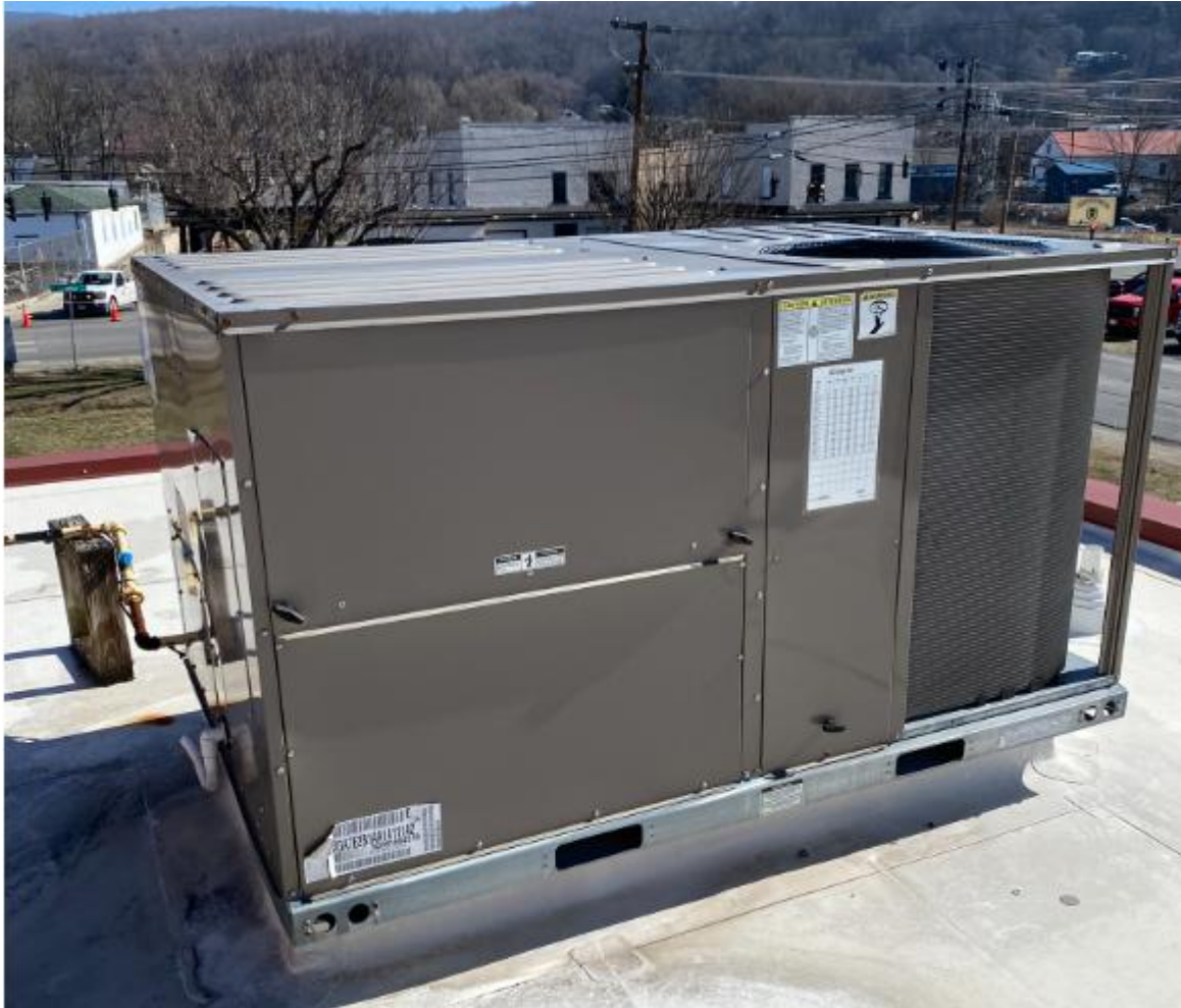
Figure 1 – Kitchen Roof Top Unit – No Outside Air Intake
