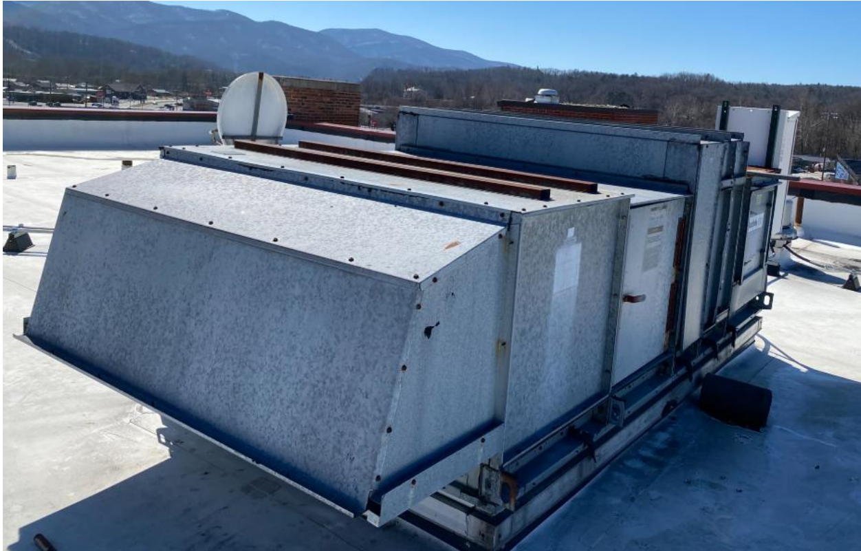
Figure 3 – Classroom RTU-4 (Dedicated Outside Air Unit). Note OA intake (at left of the unit) is approximately 40-50 feet away from the boiler stack discharge located at the far corner of the building (chimney) which is a more than sufficient distance away.
