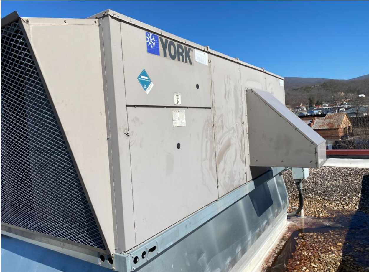
Figure 2 – Gym Roof Top Unit – with fixed, minimum Outside Air Intake Hood to the right of the unit
